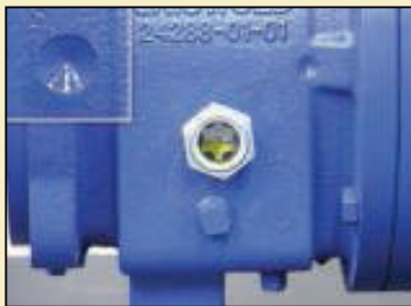
FIGURE 1. The oil level must be at the half-way point in the sight glass
